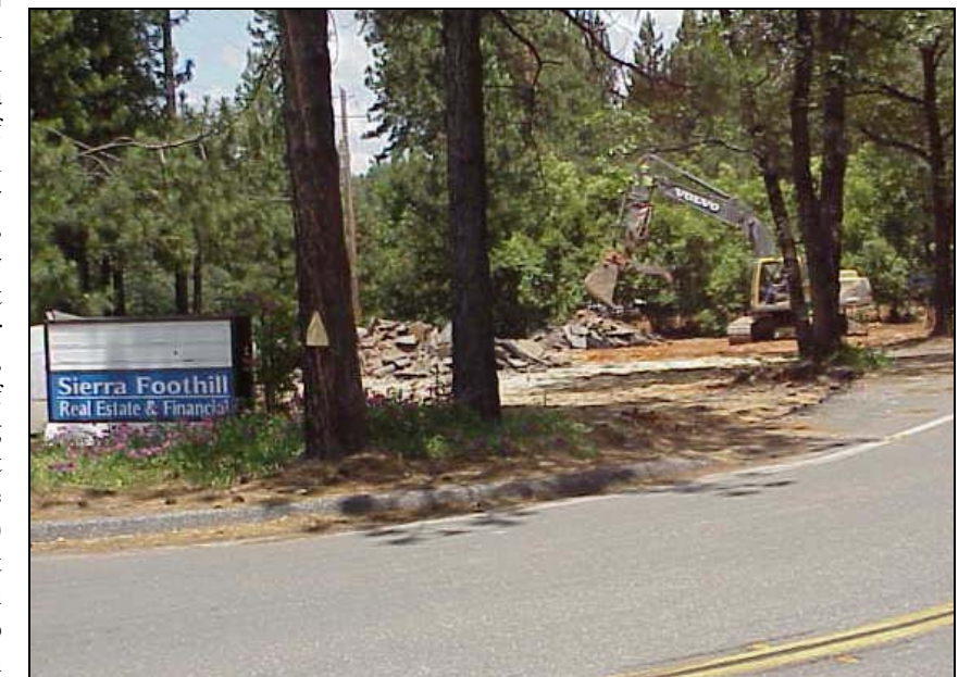
Demolition has begun on right-of-way for the La Barr Meadows Road project
